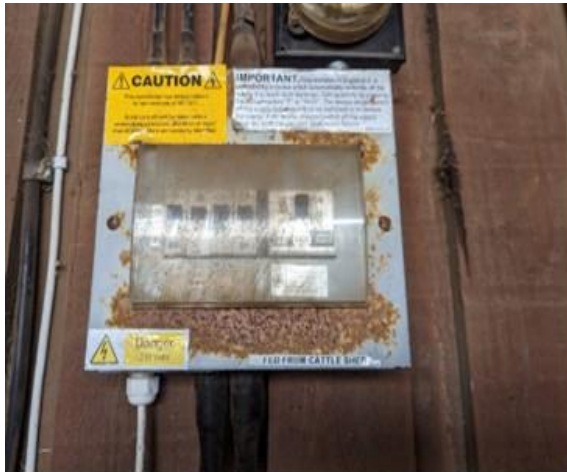
Photo 13: Machinery Shed distribution board rusted and due to be replaced.
