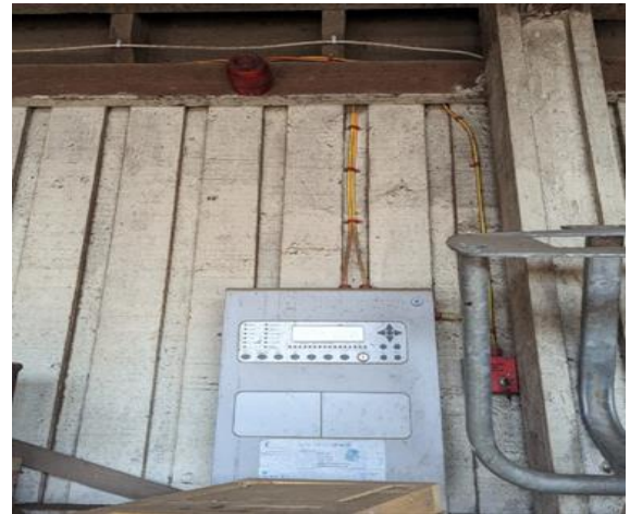
Photo 14: Non-working fire alarm panel in Machinery Shed.
