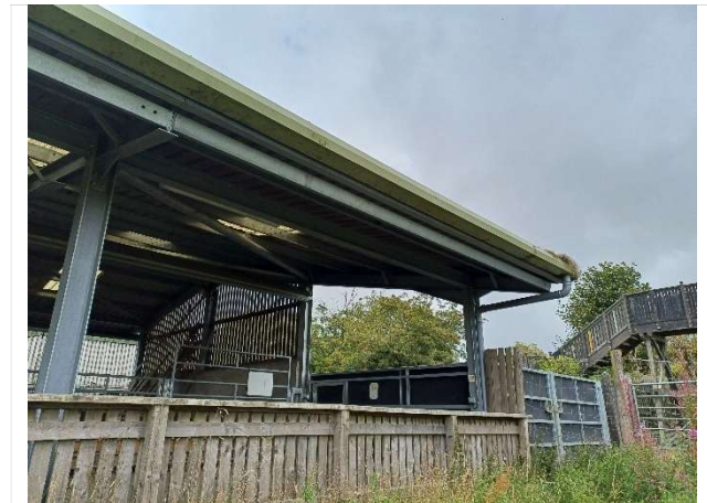
06 General view of rear elevation showing build-up of vegetation in guttering.
