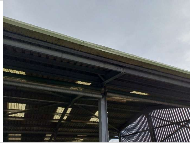
02 Dent to guttering on front elevation.
