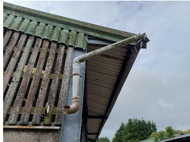
05 Poor condition of downpipe, showing missing section and discolouration highlighting possible leaks
