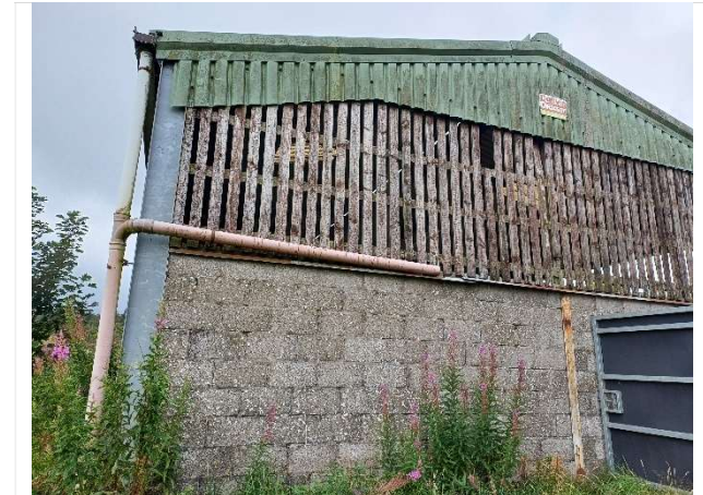
06 Second general view of left elevation showing poor condition and signs of deterioration and vegetation growth.
