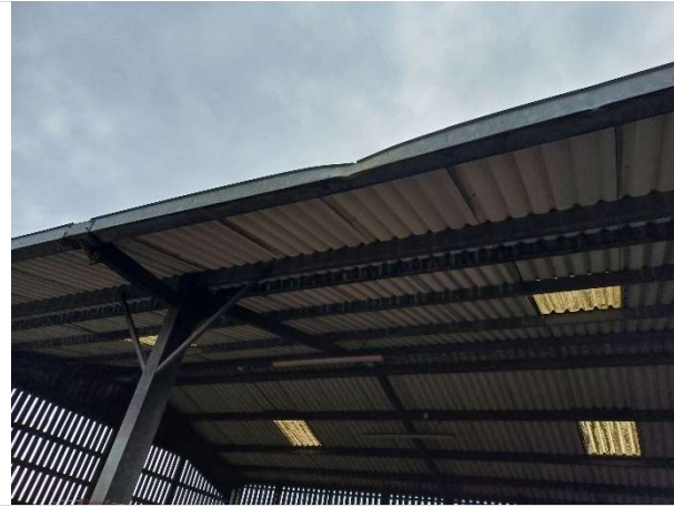
02 Damage to guttering at front elevation.
