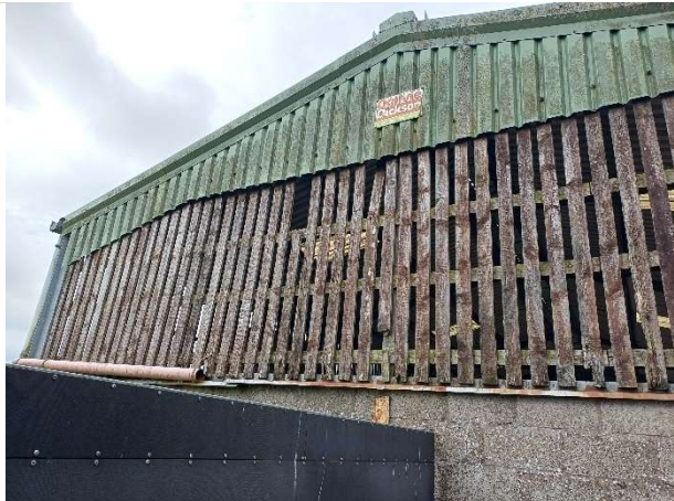
04 Metal cladding showing rust and discolouration. Section of wooden slats missing, damaged and significant deterioration.
