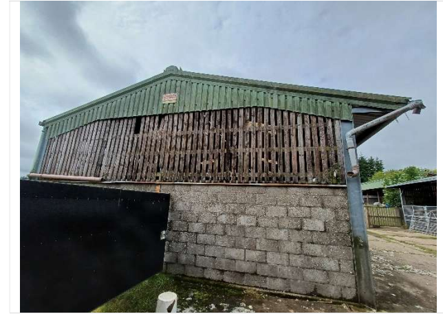
03 General view of left elevation showing poor condition and signs of deterioration.
