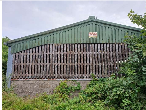
05 General view of left elevation showing weathered wooden cladding and vegetation growth.
