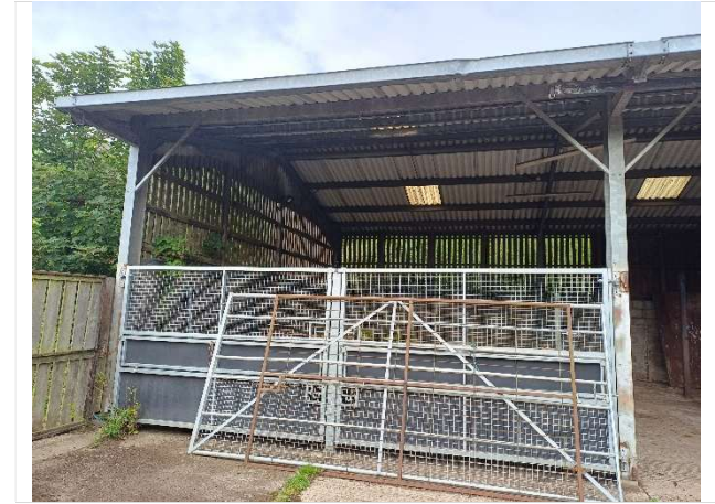
03 Minor dent in guttering to LHS of front elevation.
