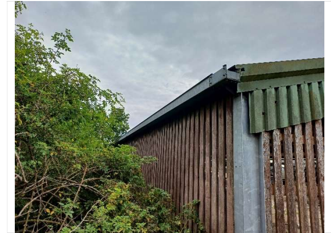
06 General view of rear elevation and guttering, showing vegetation growth.
